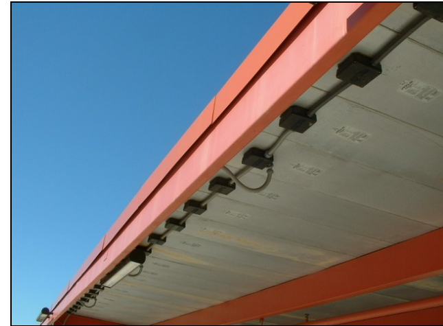
Carport solar panels
