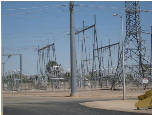
Electrical Transmission Center
