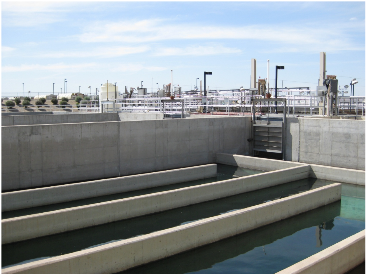
Water Reclamation Plant
