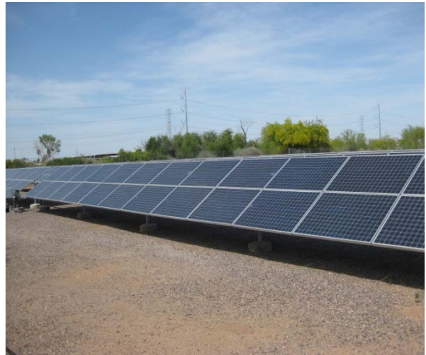
Gilbert APS Solar Power Plant
