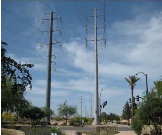
Major Power Transmission Corridor
