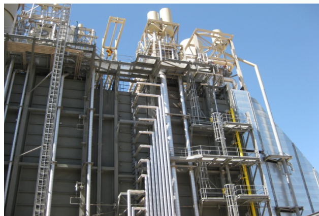
SRP Santan Generating Plant
