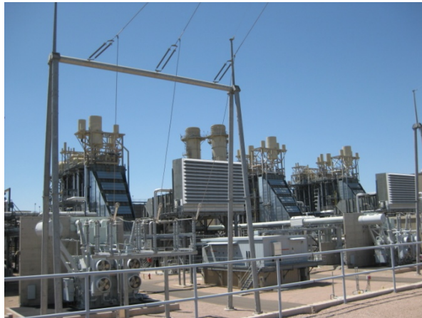
Santan Generating Plant
